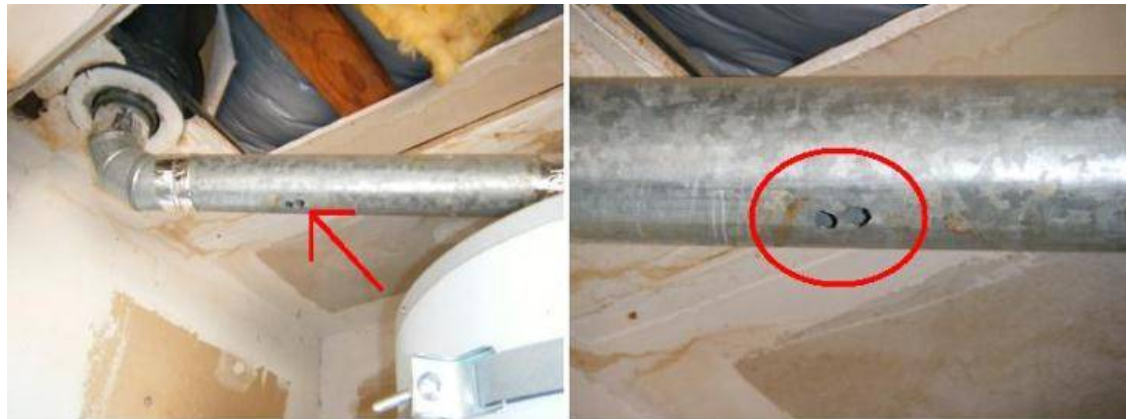
There are two holes noted in the vent.
