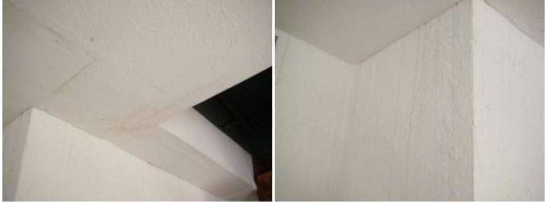
Water stains are noted in the fitness room and coming down the back side of the master bedroom fireplace.
