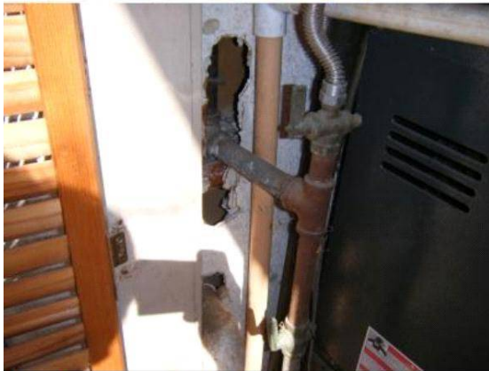
West Mechanical Room
