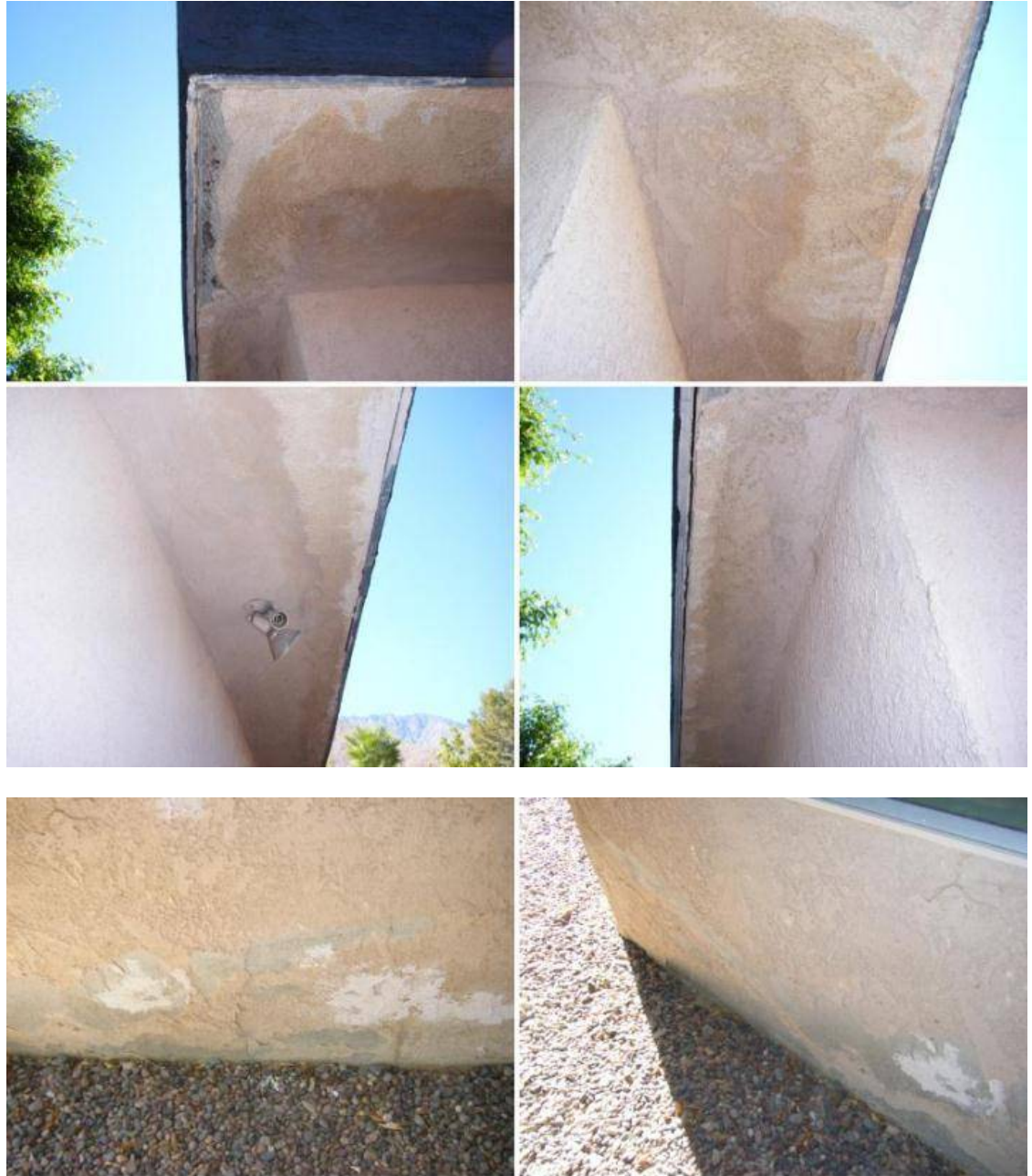
There is deteriorated color coat noted at a few section of the stucco walls.
