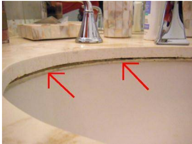
The right sink should be caulked to the counter.
