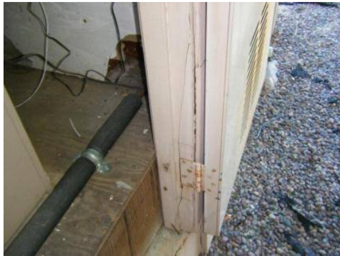
The jamb of the East mechanical closet is cracked.
